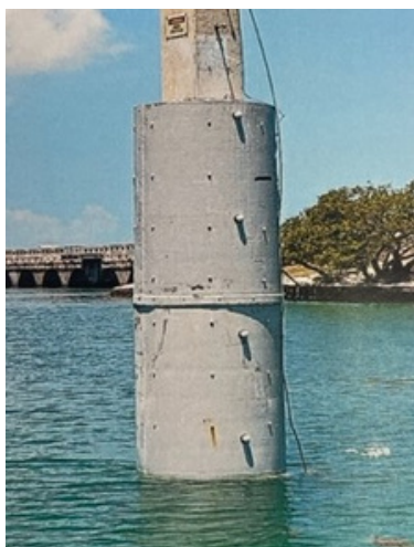
Image showing the Lifejacket Cathodic Protection System
